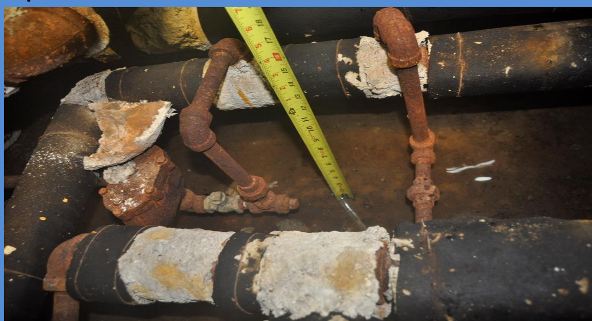
Asbestos found lining neglected pipes in the Fifth Regiment Armory
